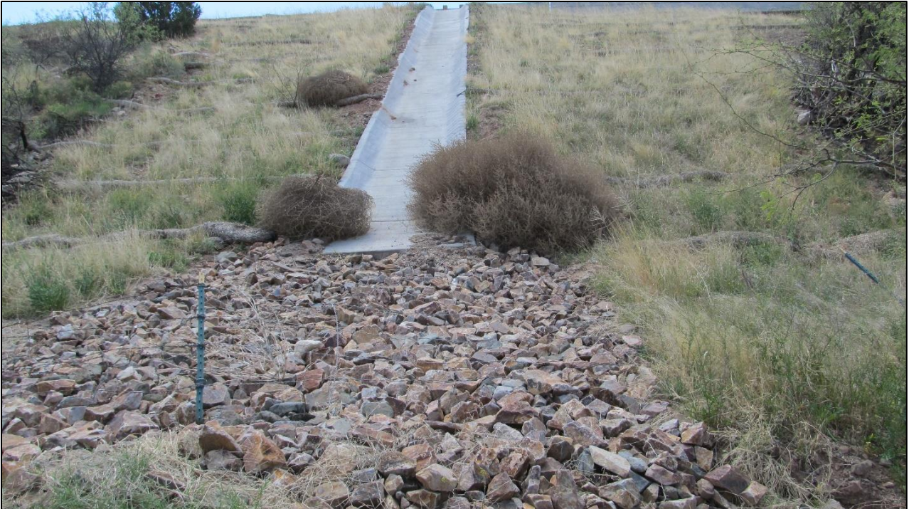
Figure 18. Photo: 3385. Fence down and in disarray.
