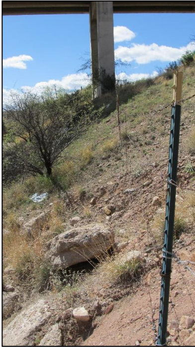
Figure 21. 3369. Insufficient fencing under bridges.
